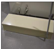
ACC20 Waste Water Trough & Pump
